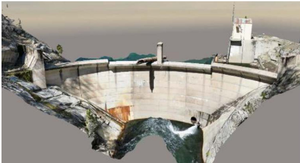
3D Image of South Fork Diversion Dam (generated from drone survey conducted by Niricson, 2022)
