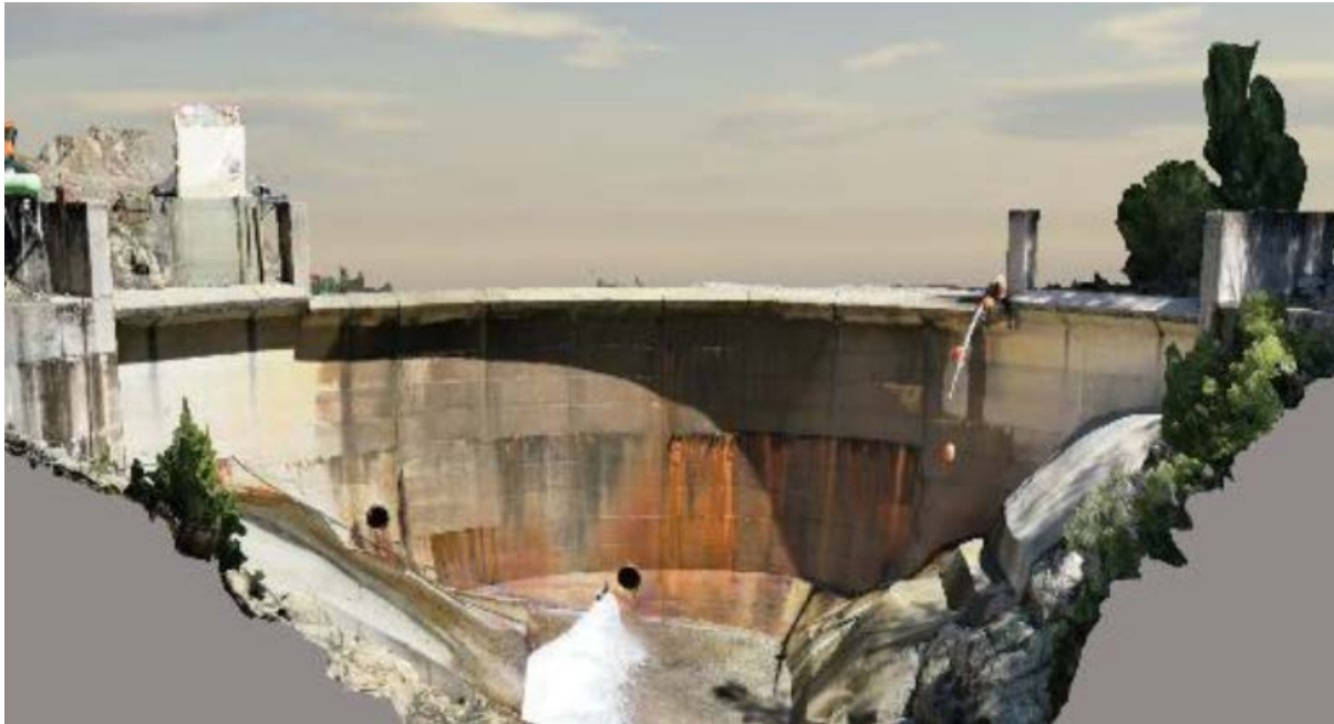
3D Image of Slate Creek Diversion Dam (generated from drone survey conducted by Niricson, 2022)
