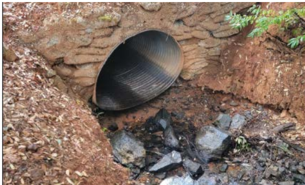
Smashed culvert pipe with gap and debris
