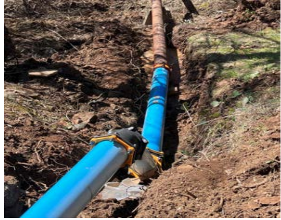
Adjoining of old and new material
