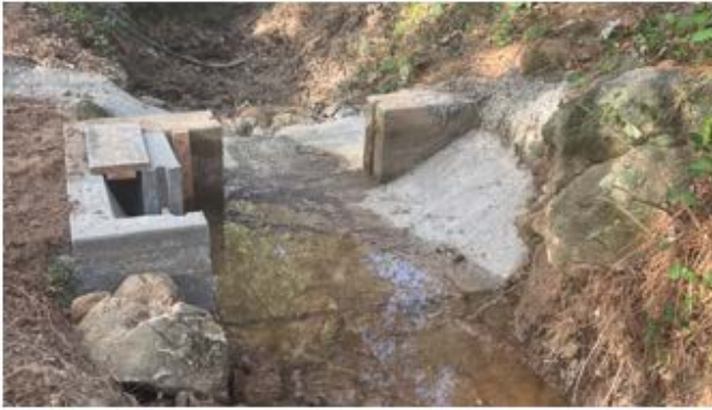
Service box repair in the South Honcut section of SFWPA's irrigation system
